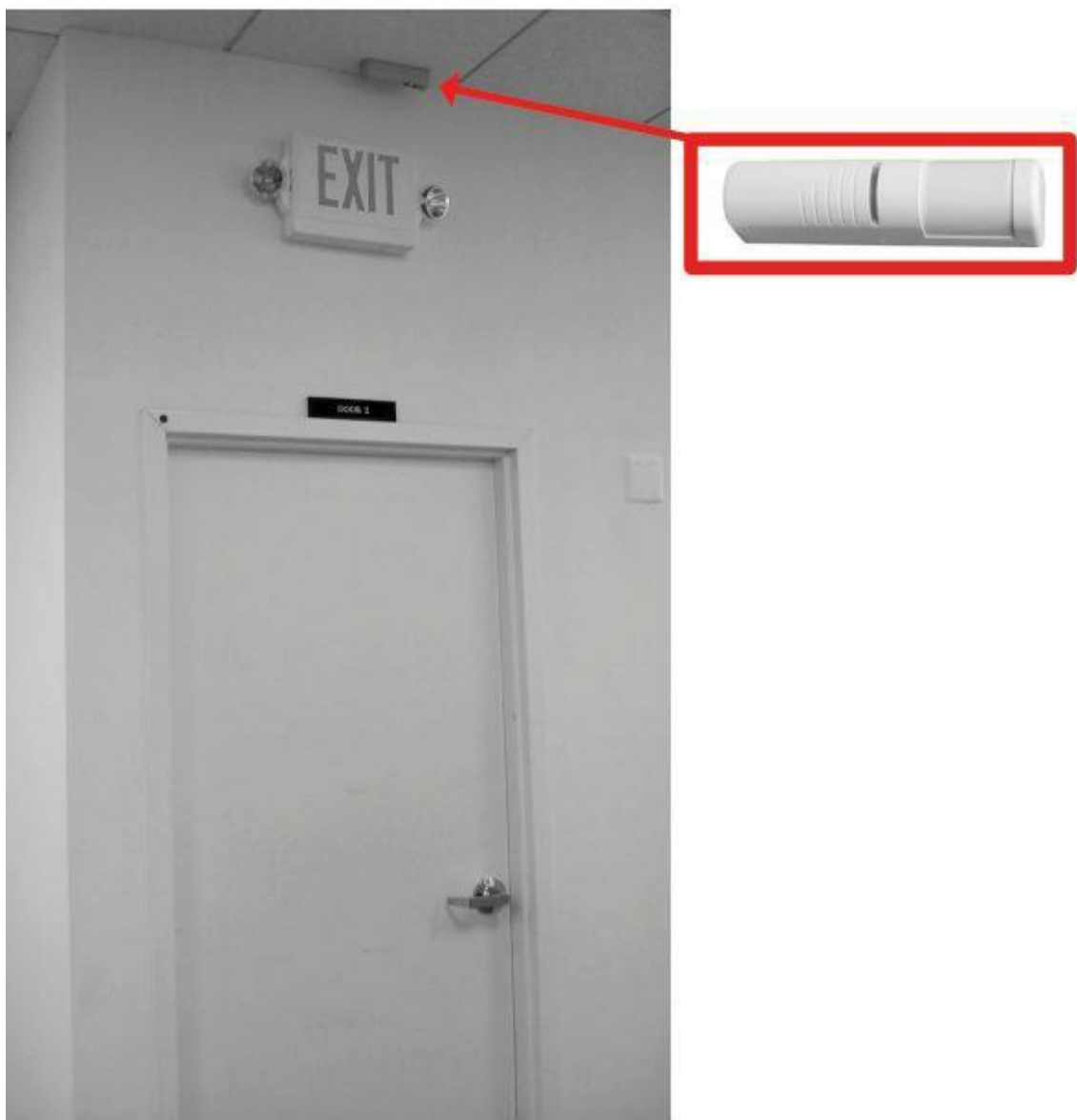
Figure 10.21 - An automatic Request to Exit (REX) device [located over the Exit sign] provides for magnetically locked doors acting as an automatic sensor for detecting an approaching person in the exit direction and deactivates the alarm as the person exits (Courtesy of Bosch Security Systems.)
