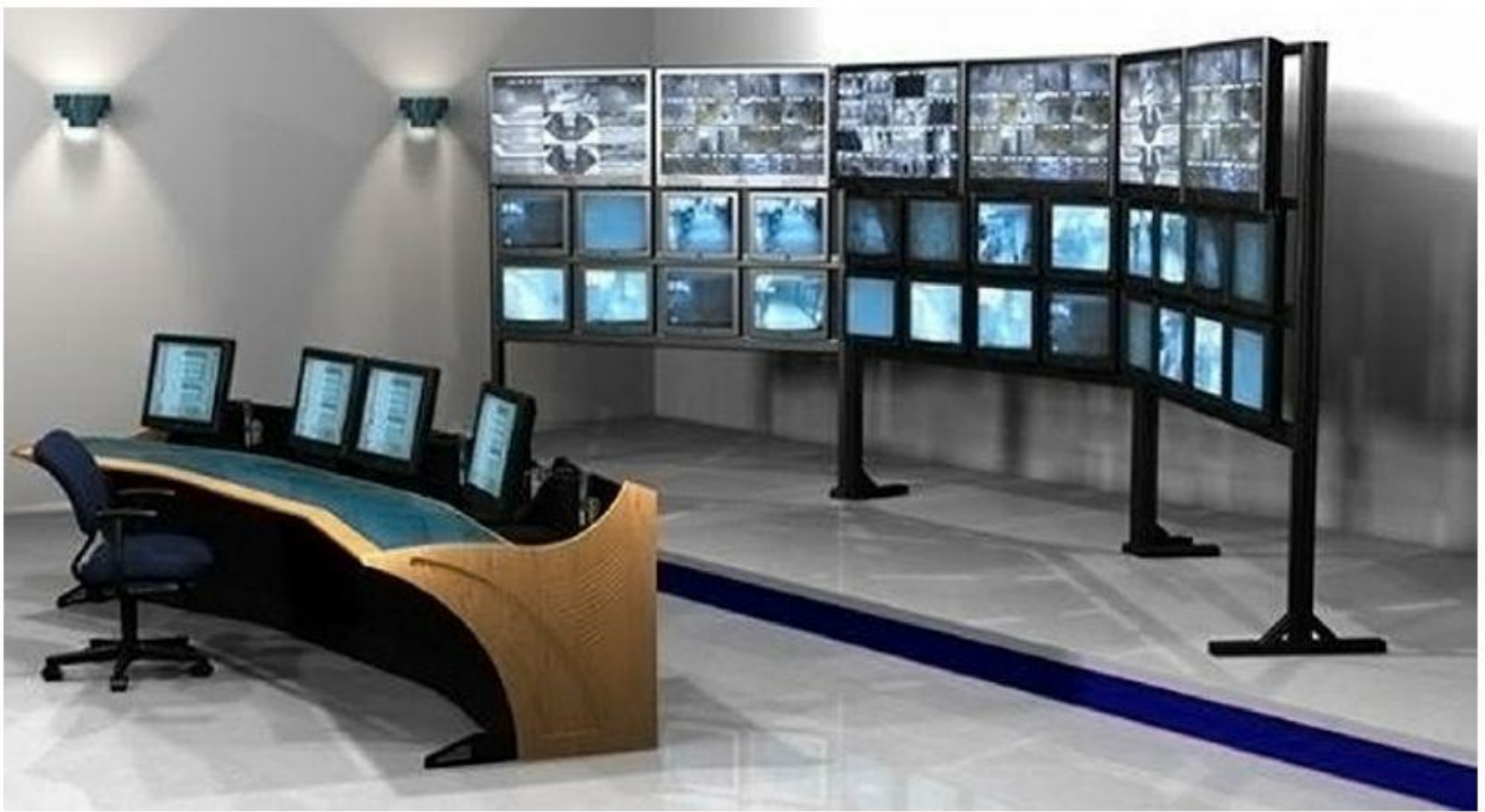
Figure 10.16 - Large Format Displays in a control center (Courtesy of Bosch Security Systems.)
