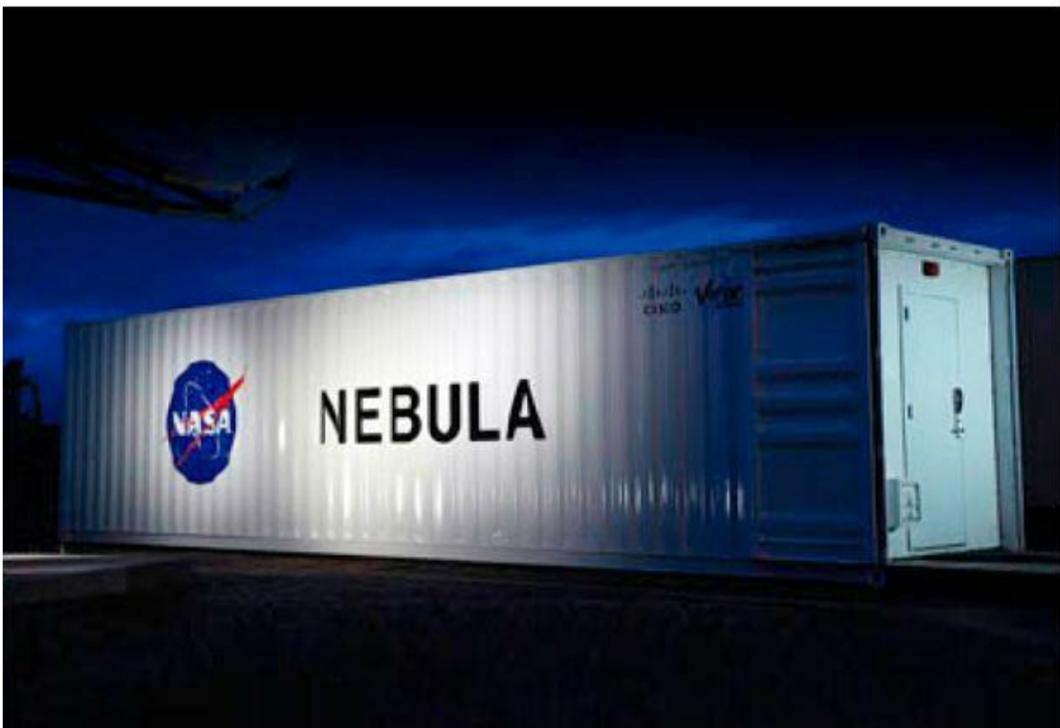
Figure 8.8 - An example of a Container Data Center module
