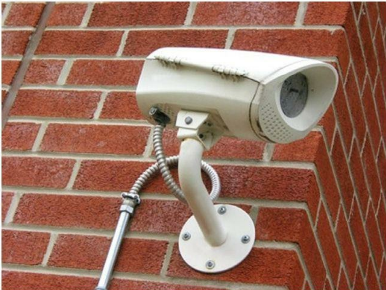
Figure 10.13 - A Wall-Mounted Camera (Courtesy of Bosch Security Systems.)
